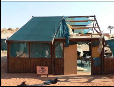
NaDEET Centre after the fire
