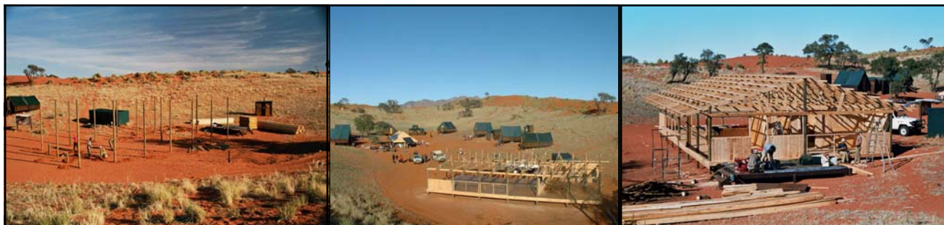
1. Planting the poles 2. View of NaDEET Centre with tented classroom & half finished main building 3. Starting on the side walls
